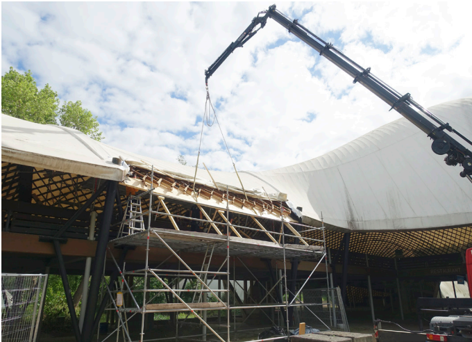
Figures 8: Images of the initial trial repair phase (completed in 2024), which included three test areas to gain a better understanding of the optimal renovation process. The exchanged and reinforced slats are clearly visible; the replacement of the roof covering membrane. Images by Fast + Epp (2024).
