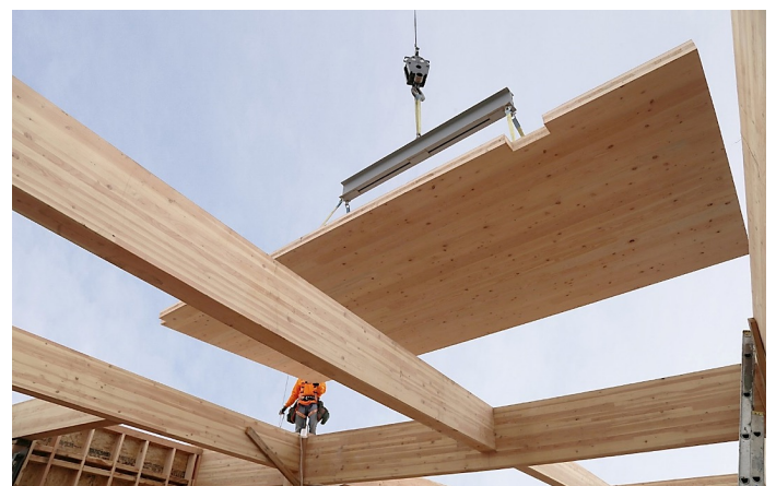
Figure 1: A lightweight CLT panel is hoisted into position: a mass timber construction project in the US, using CLT panels and glulam beams (courtesy of Lever Architecture, 2023).
