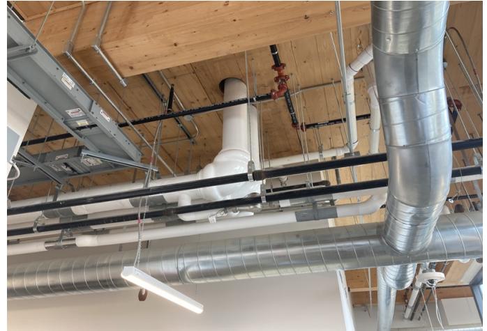
Figure 3: Overhead MEPFP Systems
